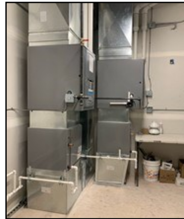
Photo above: Phase II Mechanical Room.
