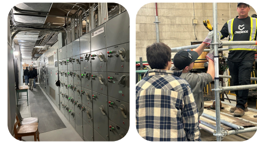
Pictured above: Chad Rennie presents a tour of the YRHS Electrical system and Credence Construction presents a scaffolding demonstration.
